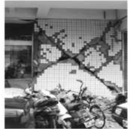
Figure 2-20 Typical infill wall diagonal crack pattern, 1999 Chi-chi, Taiwan earthquake. (Reproduced with permission from Geoff Sawell).
