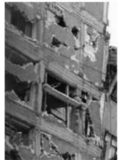
Figure 2-21 Damage to the tops of several columns due to infill wall compressive strut action, Mexico City, 1985 Mexico earthquake. (Reproduced with permission from R.S. Shephard).
