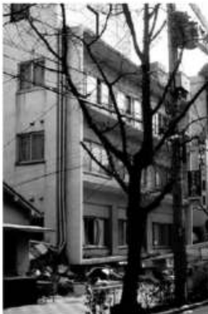
Figure 2-2 Soft storey ground floor collapse of a four-storey building. 1995 Kobe earthquake. (Bertero, V.V. Courtesy of the National Information Service for Earthquake Engineering, EERC, University of California, Berkeley).
