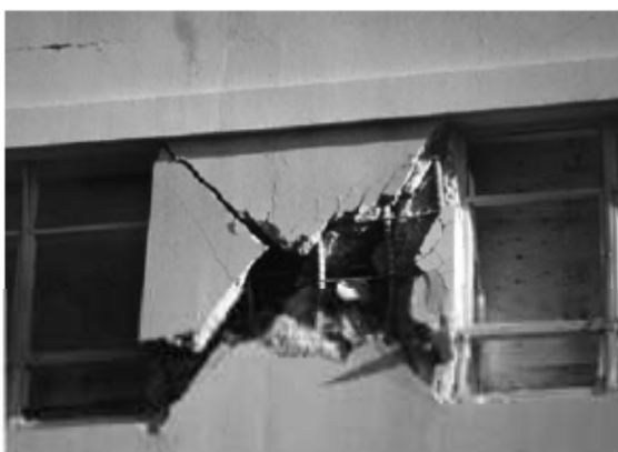
Figure 2-11 Typical short column damage. 1994 Northridge, California earthquake. (Reproduced with permission from Andrew B. King)
