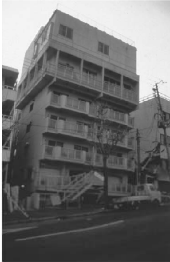
Figure 1-5 Collapse of a concrete frame building at ground floor level due to torsion, 1995 Kobe, Japan earthquake. (Reproduced with permission from EERI, David R. Bonneville, photographer)
