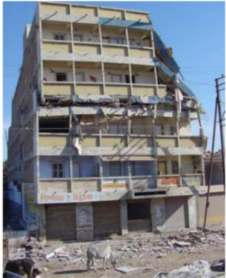
Figure 2-6 C Collapse of soft middle storey in a building at Bhuj.
