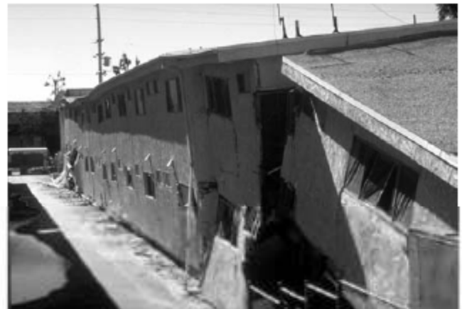
Figure 2-1 A soft storey ground floor has disappeared in this three-storey apartment block. 1994 Northridge, California earthquake. (Jetherran, R.K. Courtesy of the National Information Service for Earthquake Engineering, EERC, University of California, Berkeley).
