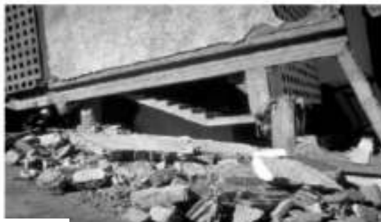
Figure 2-16 Ground floor damage caused by a discontinuous wall. 1980 El Asnam, Algeria earthquake. (Bertero, V.V. Courtesy of the National Information Service for Earthquake Engineering, EERC, University of California, Berkeley)
