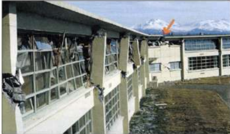
Figure 1-13 West Anchorage High School, Alaska earthquake, 1964. Stress concentration at the notch of this shallow L-shaped building damaged the concrete roof diaphragm.
